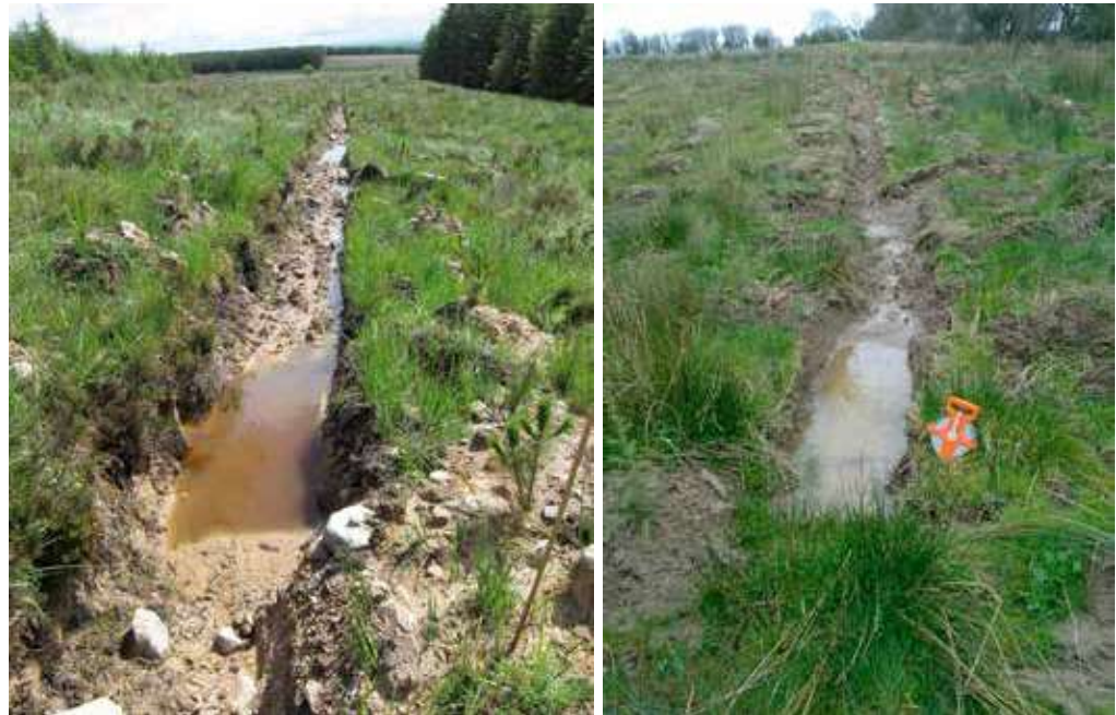
In-drain sediment trap (left) and a sediment trap adjoining a water setback (foreground) (right).
